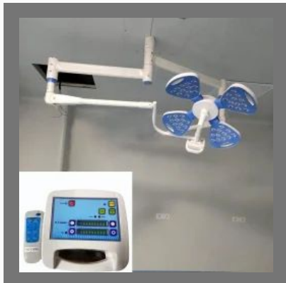
Single Ceiling Dome LED OT Light
